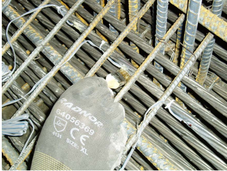
Figure 6-21: Application of the epoxy resin (the first layer of coating) over a FLA-5-11-5LT strain gage mounted on a vertical leg of a typical No.5 end zone rebar.
